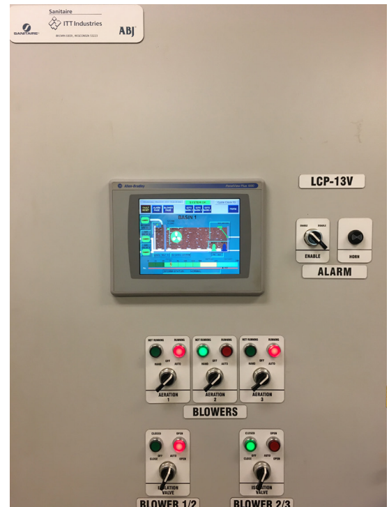
Former HMI hardware and software mounted in the existing control panel
