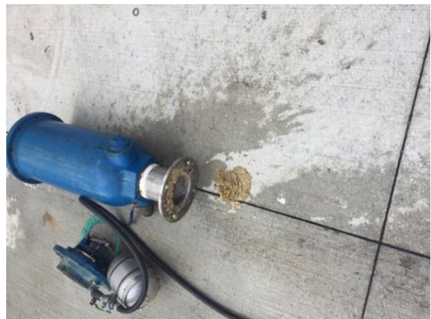
Photo from Air valve cleaning 19 th March, 9 days after WW installation. This is the typical 'Post-WWW' FOG removed from the valve
