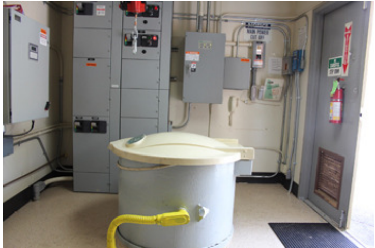
This underground lift station by S&L has been in operation for 40 years
