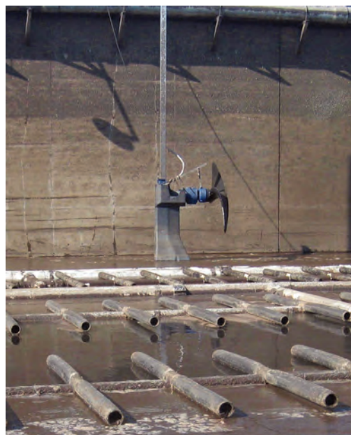
Fig. #24 - Combined Mixing & Aeration
