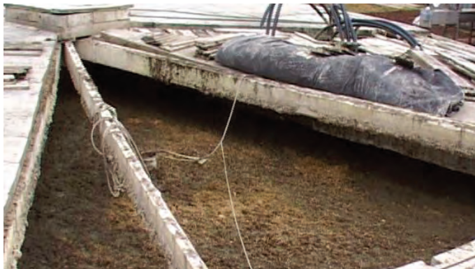
Fig. #10 - Anaerobic Digester Sludge - No Mixing
