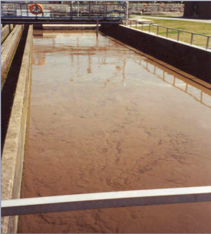
Fig. #43 - Poor mixing in long tank
