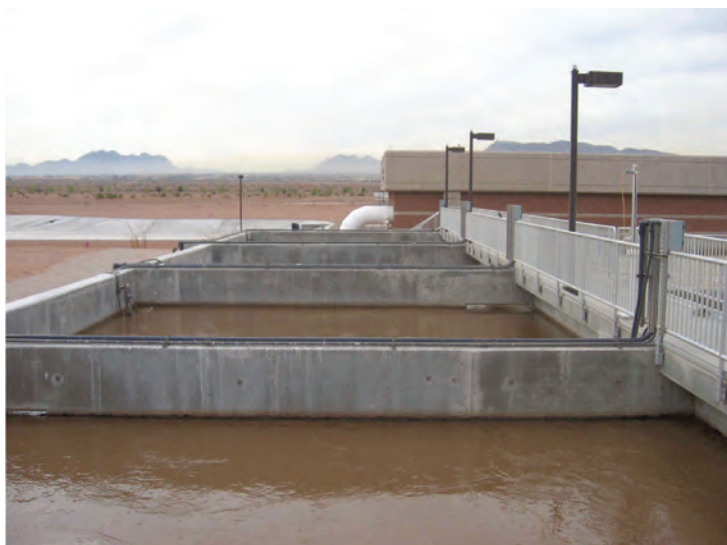
Fig. #1 - Typical WWTP Process Tank (Henderson, NV)
