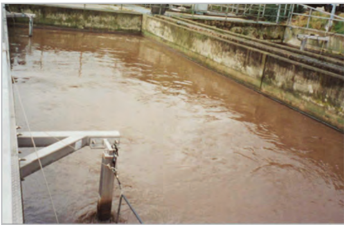
Fig. #44 - Good mixing in long tank
