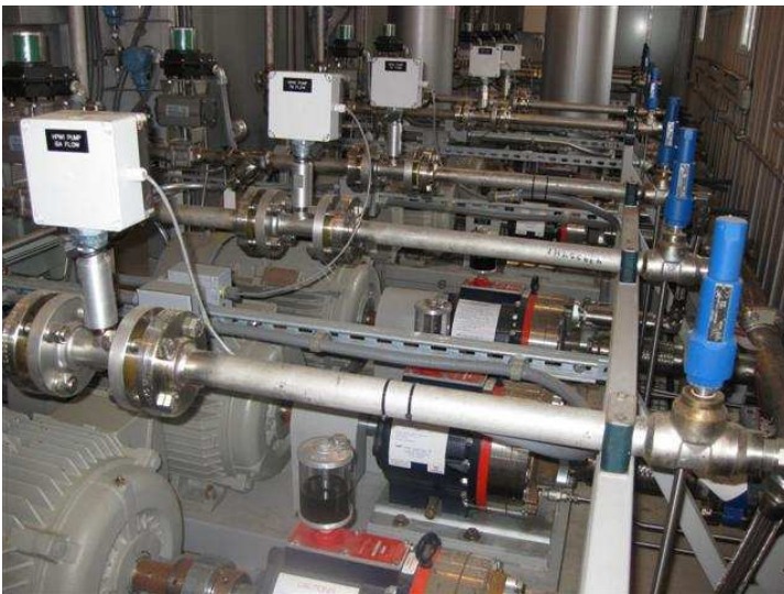
Figure 2. New high-pressure water injection system significantly cuts NOx emissions.
