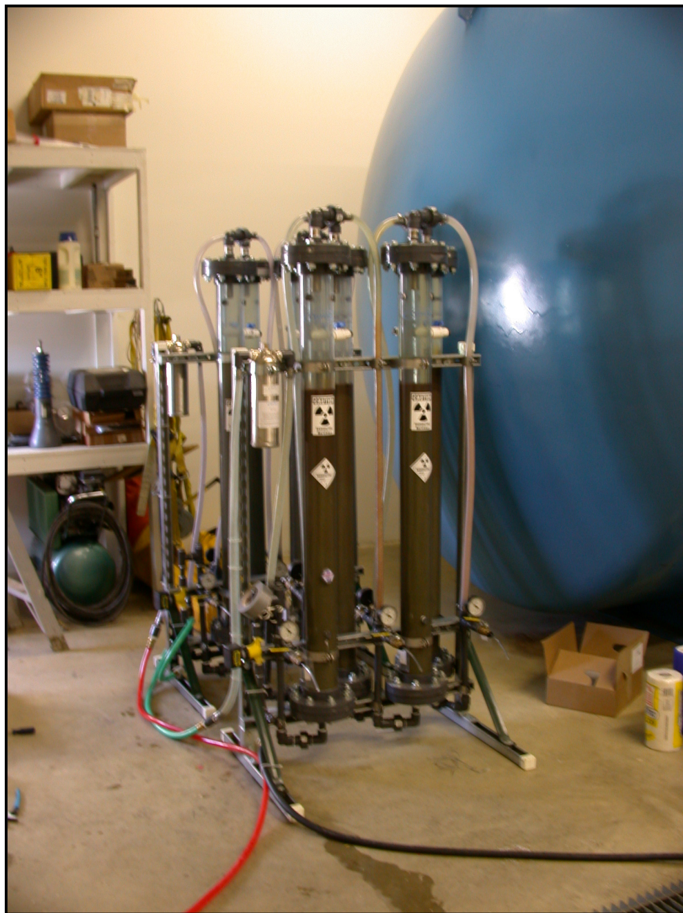
Pilot unit in operation at the Wynstone Property Owners Association
