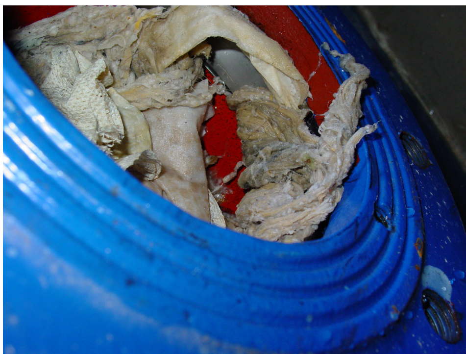
Example of a pump loaded with wipes
