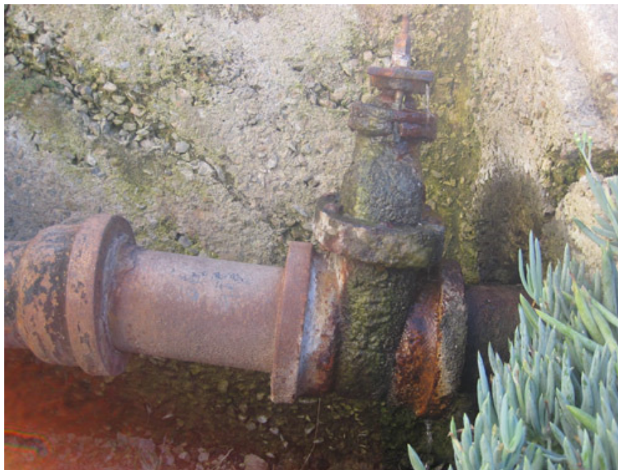
Antiquated leaking valve on Catalina Island, California
