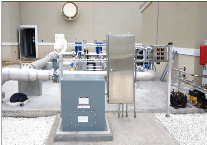
Figure 3 - Pinnacle Ozone injector process trains in late 2014.
