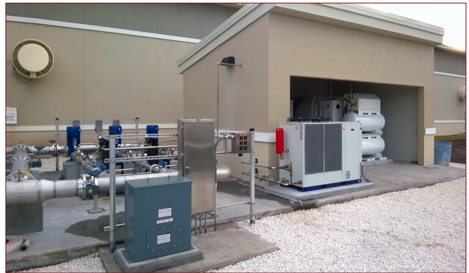
Figure 4 - Process trains, chiller, VSA O_2 , and ozone building.
