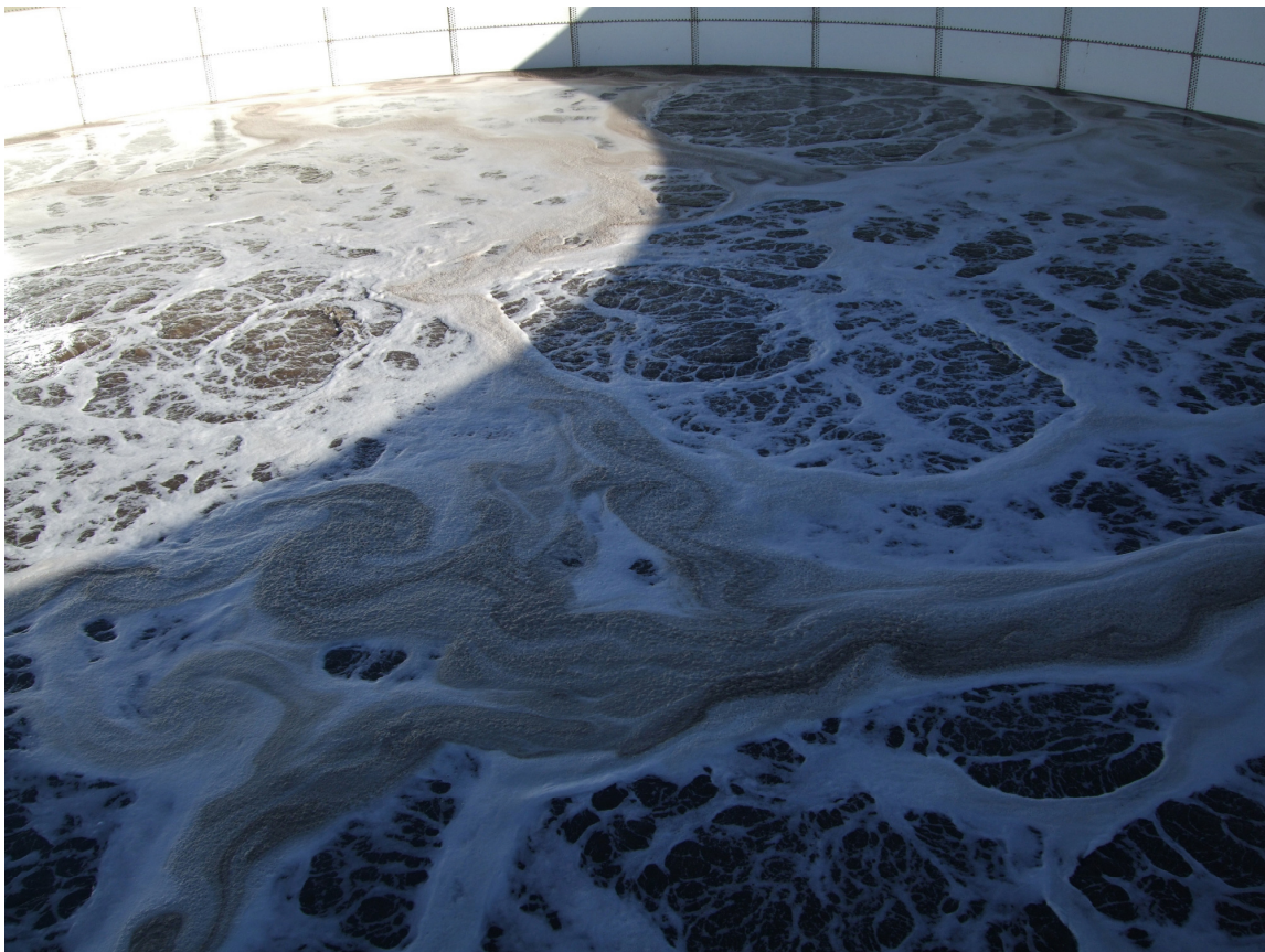
Slot Injector System - Surface Aeration Pattern
