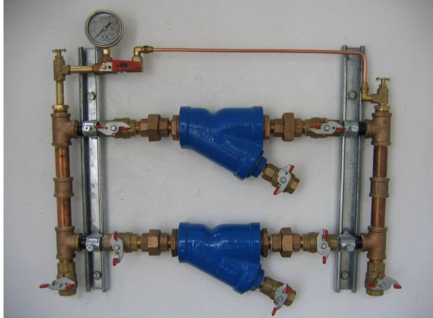
Duplex strainer set up with built in manual redundancy.
