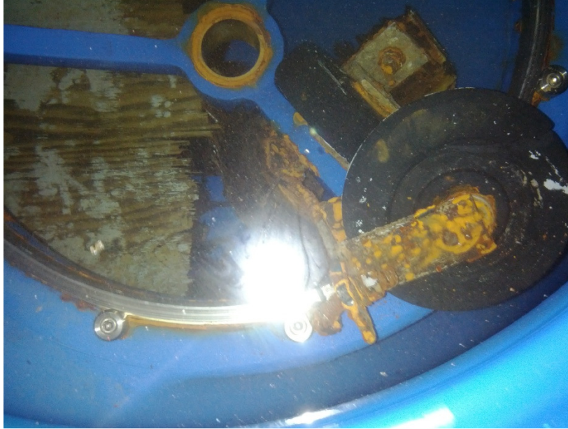
Photo of an inspection creeper or cart that was not removed from pipeline before commissioning and pressurizing the line. Again caught in the seat area of the valve, resulting in valve failure, California, USA.
