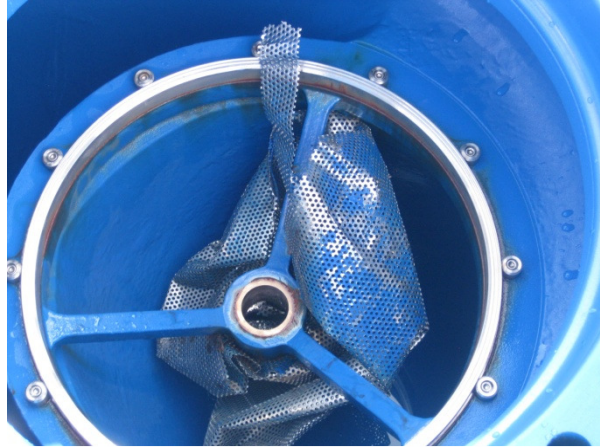
Example of debris being lodged in the lower guide and seat area of the ACV, Hail, Saudi Arabia
