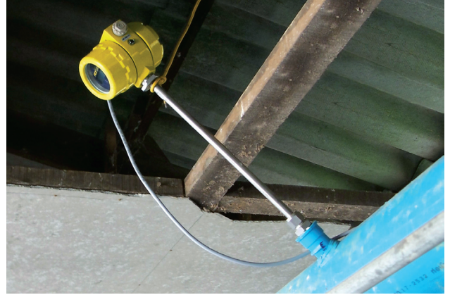
Figure 4: Flow meters installed in S.P.M. (roof interior with pipe run and meters)
